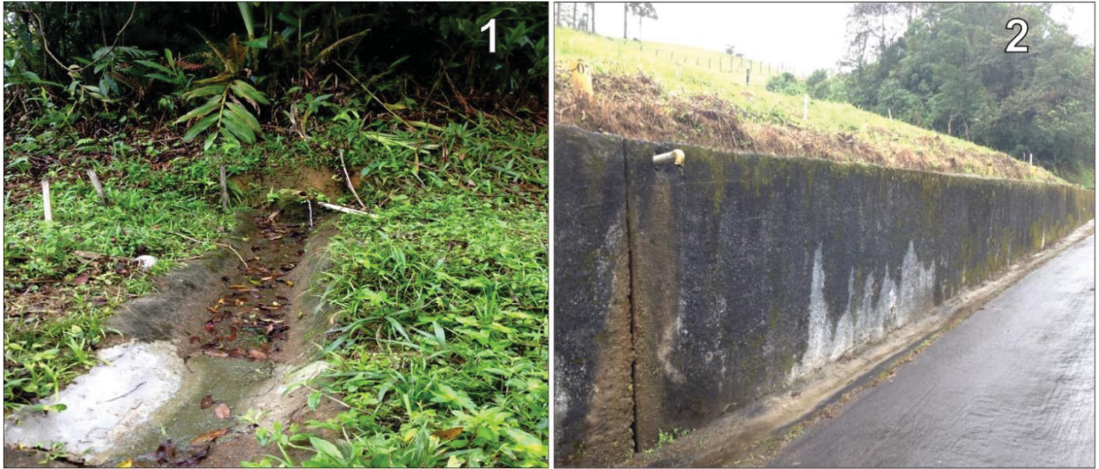
Figure 9: 1) Groundwater upwelling point; 2) Soil water logging zone.
