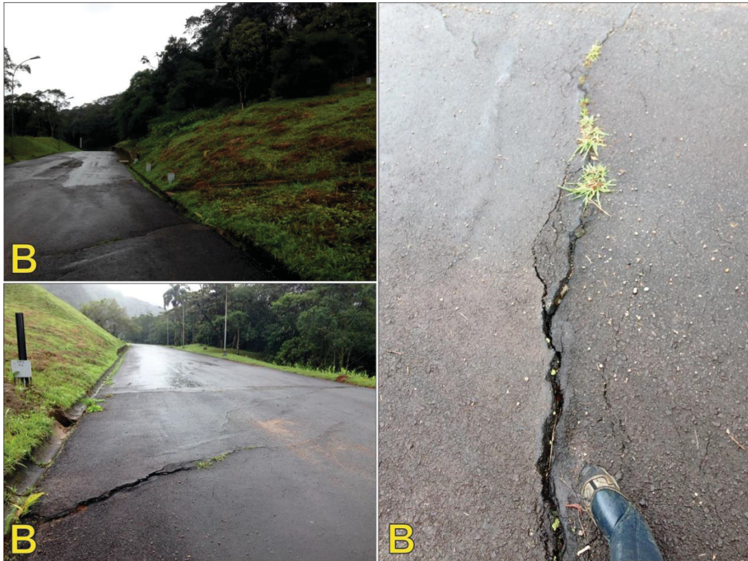
Figure 7: Tension cracks on the roadbed adjacent to the wall.
