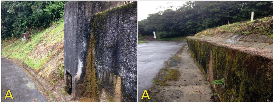
Figure 6: Broken retaining wall in the way situated at the foot of the slope considered critical point.
